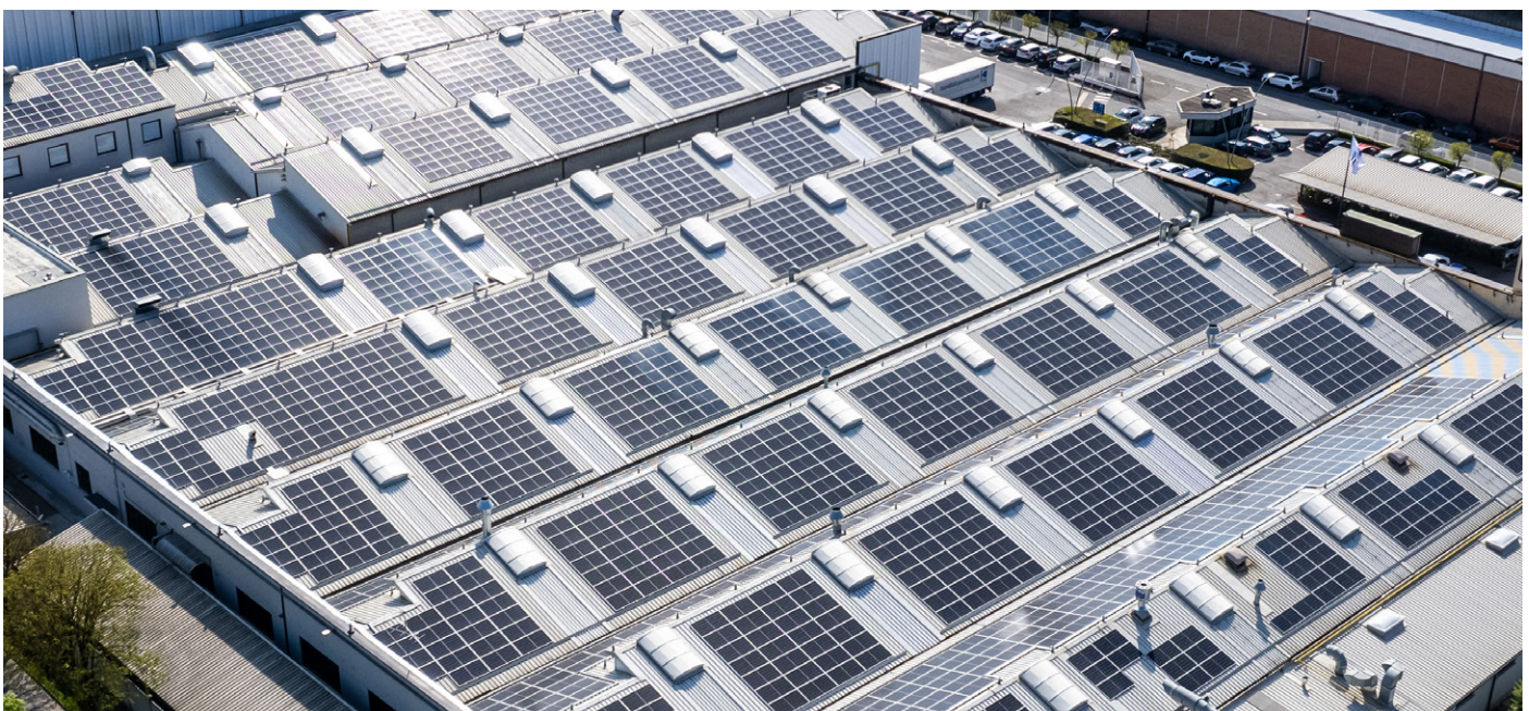
Detail of the photovoltaic plant at the main Headquarters (Suzzara, 2023)
